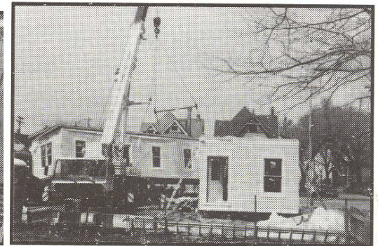
Modules are set on the foundation with a crane in one day.
